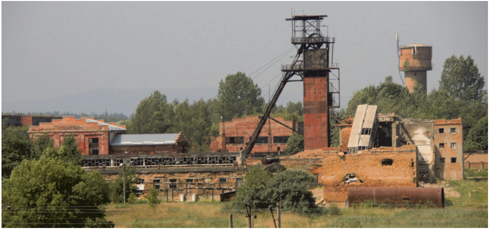
Fig. 4. Ruined and useless post-mining facilities in Stebnik, Ukraine, the relics of a liquidated salt mine
